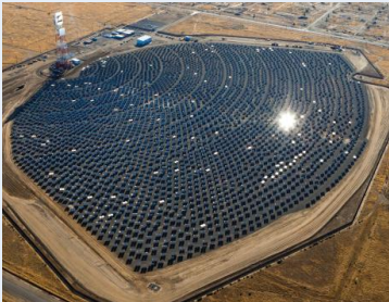
Coalinga (CA) 29 MW thermal Chevron-BrighSource Solar to Steam Demonstration Facility
